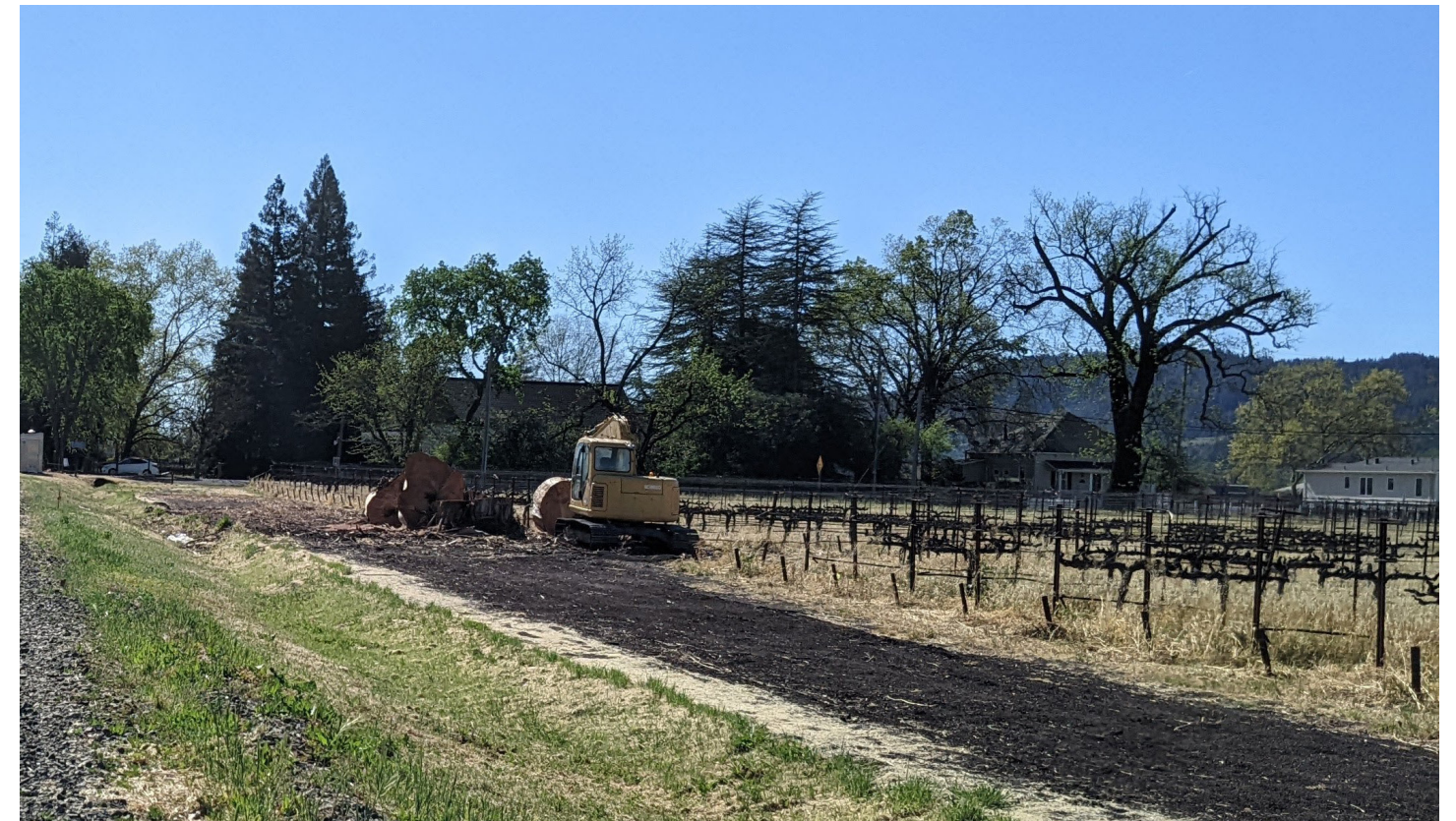
Agricultural roads at the end of vineyards are critical for ongoing operations
